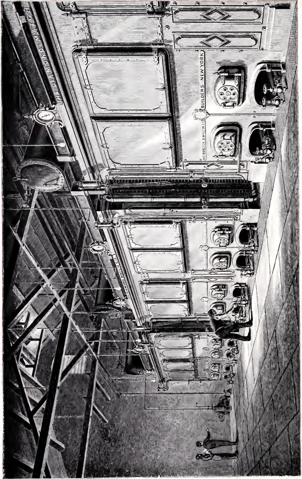
Babcock & Wilcox Boilers at Wabash Paper Co. Wabash, Ind., with Hoppe Feedwater Purifiers. 1,250 H. P. Erected 1889.
